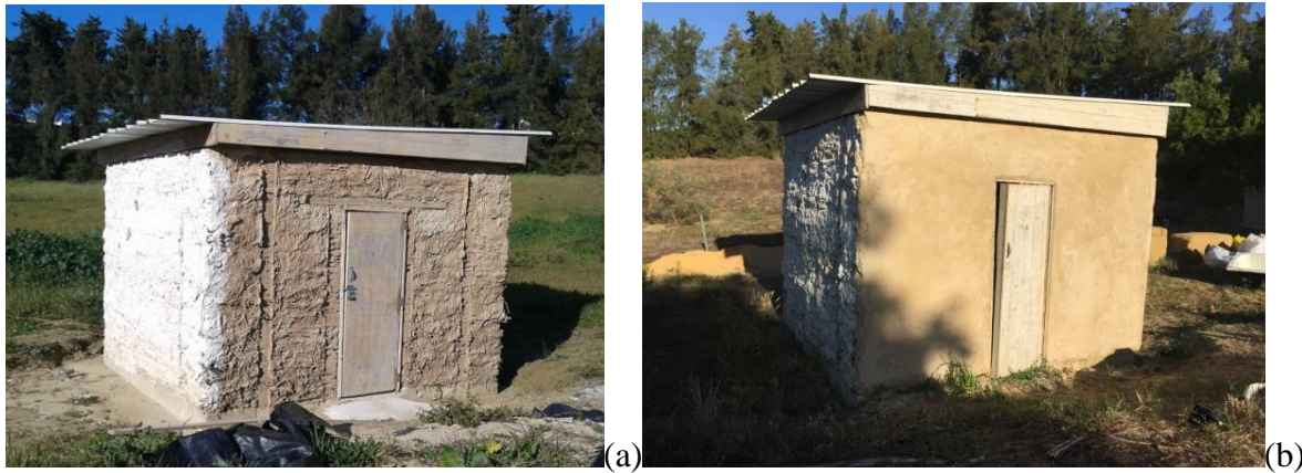
Figure 6-6 Reed-cob experimental cellule: a) shortly after construction with unrendered walls and b) five years after construction during the application of a protective render on the wall surface.
