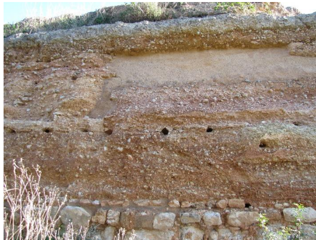
Figure 6-5 Erosion at the base of a rammed earth wall in Paderne Castle, Portugal.
