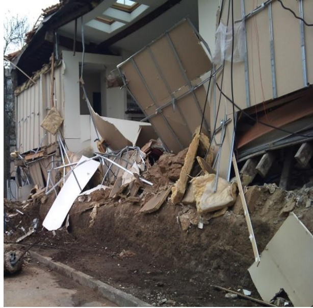
Figure 6-1 Collapse of an earth building in Lyon, France, due to the accumulation of humidity at the wall base.
