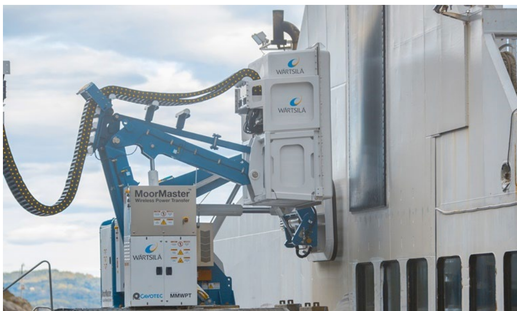
Figure 5. The world's first automatic wireless induction charging system on Norled's hybrid ferry, developed by Wartsila [94]. Credit: Shippax.
