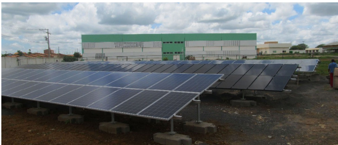
FIGURE 5 IFBA's reference photovoltaic plant linked to the project "Development and testing of systems for photovoltaic solar generation in high-temperature conditions in semi-arid regions of northeastern Brazil." 35
